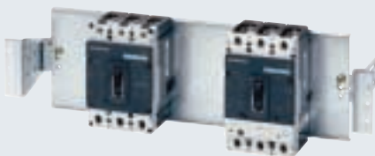
Outgoing feeders with 3VL circuit-breakers fixed on a mounting plate
