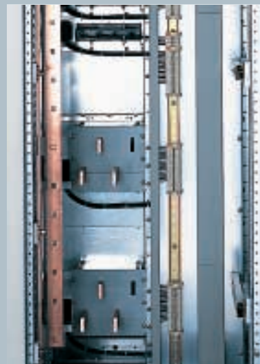
Cable connection rear
